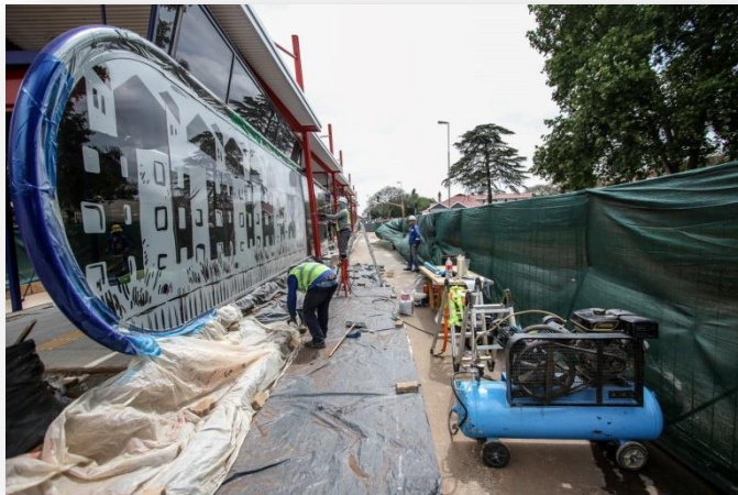
Example Reya Vaya Artworks: The KES Station along the Louis Botha Corridor. The sandblasted design is against the glass panel.
